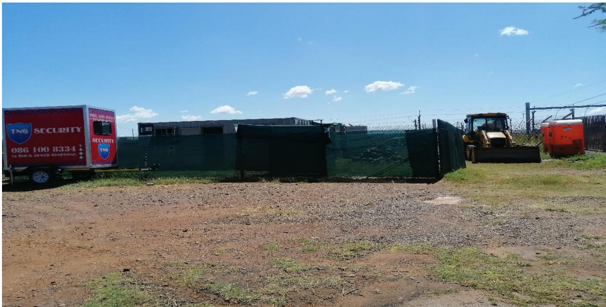
Figure 4: Security / guard post and chemical ablution facilities in substation site camp.
